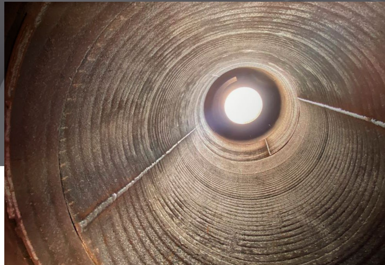
Internal cyclone with DAIKOPLATE 640 sheet
